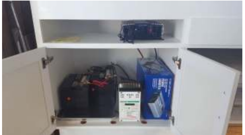
Two 12 volt Batteries stored in New Cabinet
